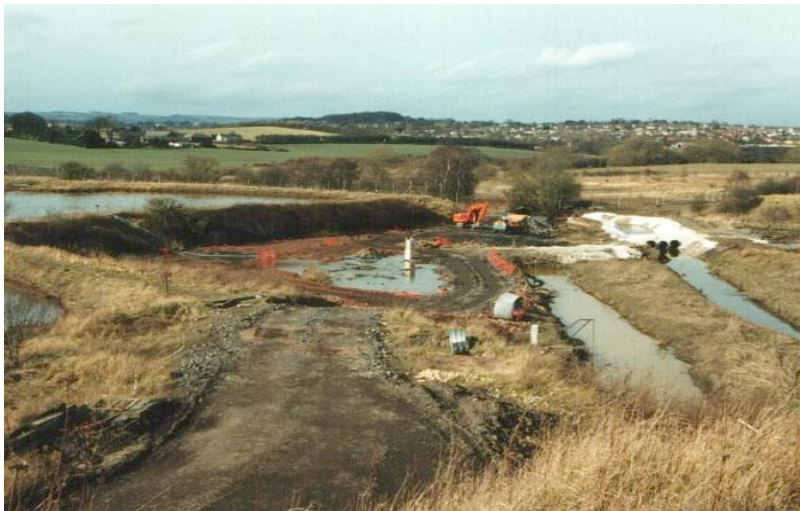
Contaminated Site, East Midlands, UK
